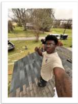
Winner Banissan showing the work done on a roof during his spring break mission trip to Cary, Mississippi.
